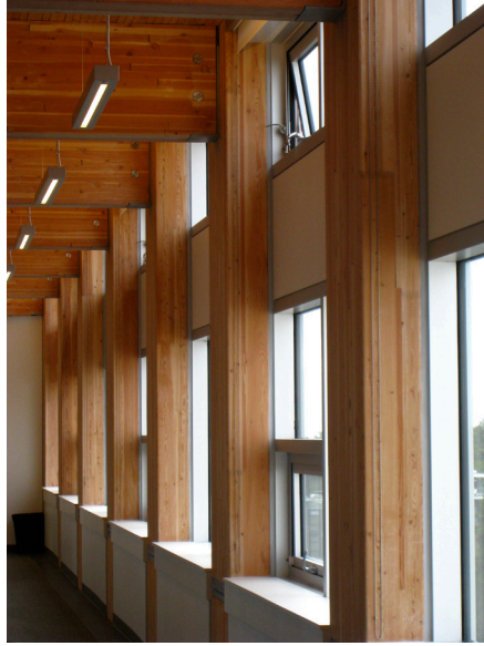
Image 9.2 Glue-laminated beams in structural moment frames. Photograph by Martin Tessler.
